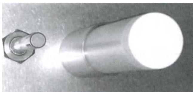
Figure: Installed CO 2 sensor (right) and CO 2 mixing head
