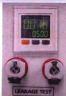
Leakage test fittings (pressure indicator and test setting)
