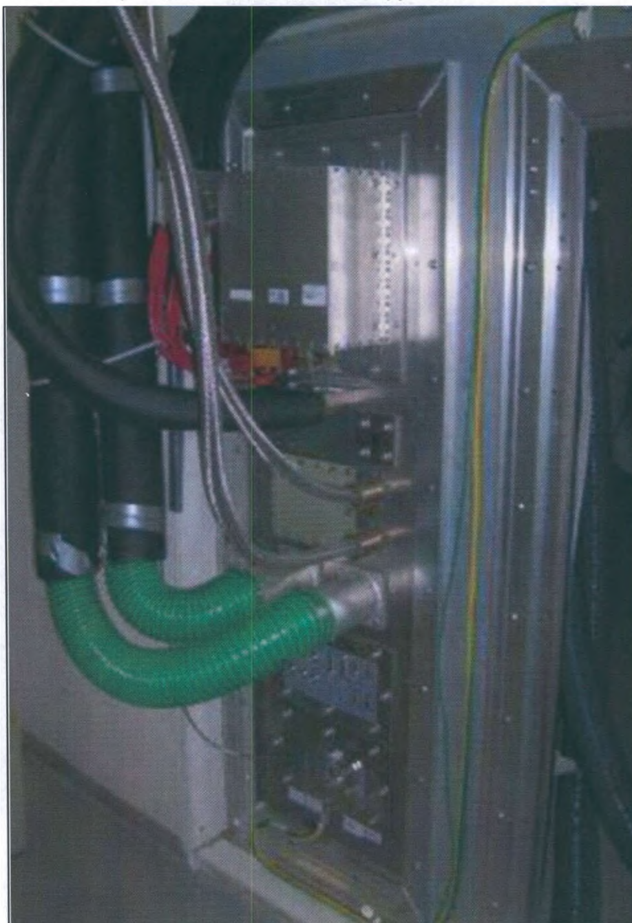
Scan Room Side
