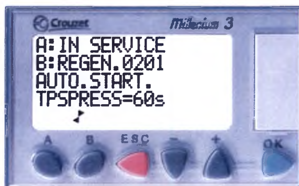
Figure 13 – Dryer control unit (Millenium 3)
