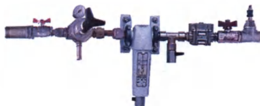
Figure 8 – Pressure reduction line at 8 bar, (as the example of model DP 217 S) external view
