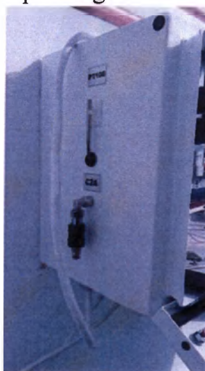
Figure 20 – Left side of control unit Cyclic 2020
