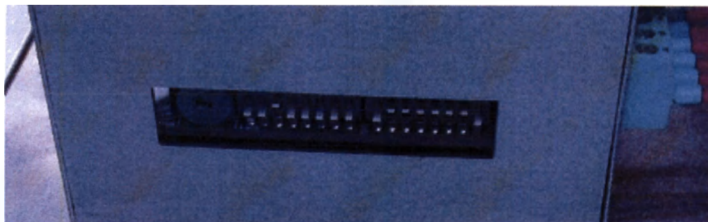
Figure 24 – SW switchers in a control unit
